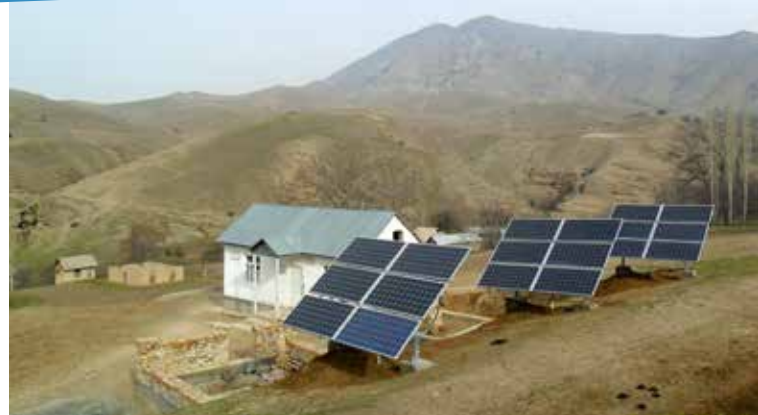
3 kWt photovoltaic station, installed by UNIDO at the First Aid Station (FAS) in Tashtak village, Akсы district, Jalal-Abad province in March 2013. The FAS serves 1080 people.
